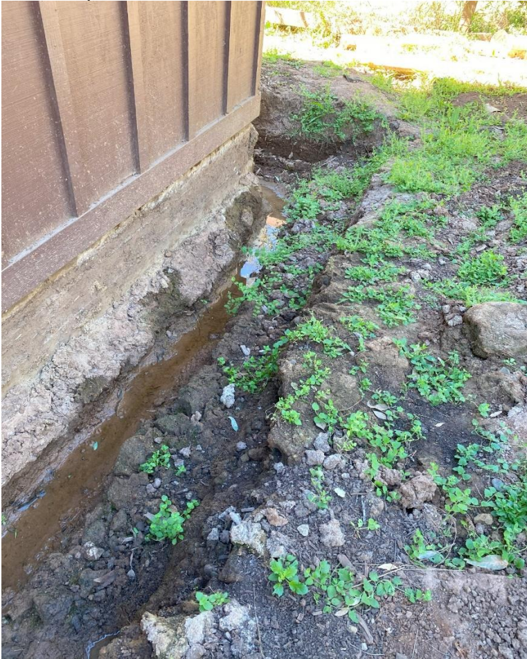
Early October water seepage continued.
