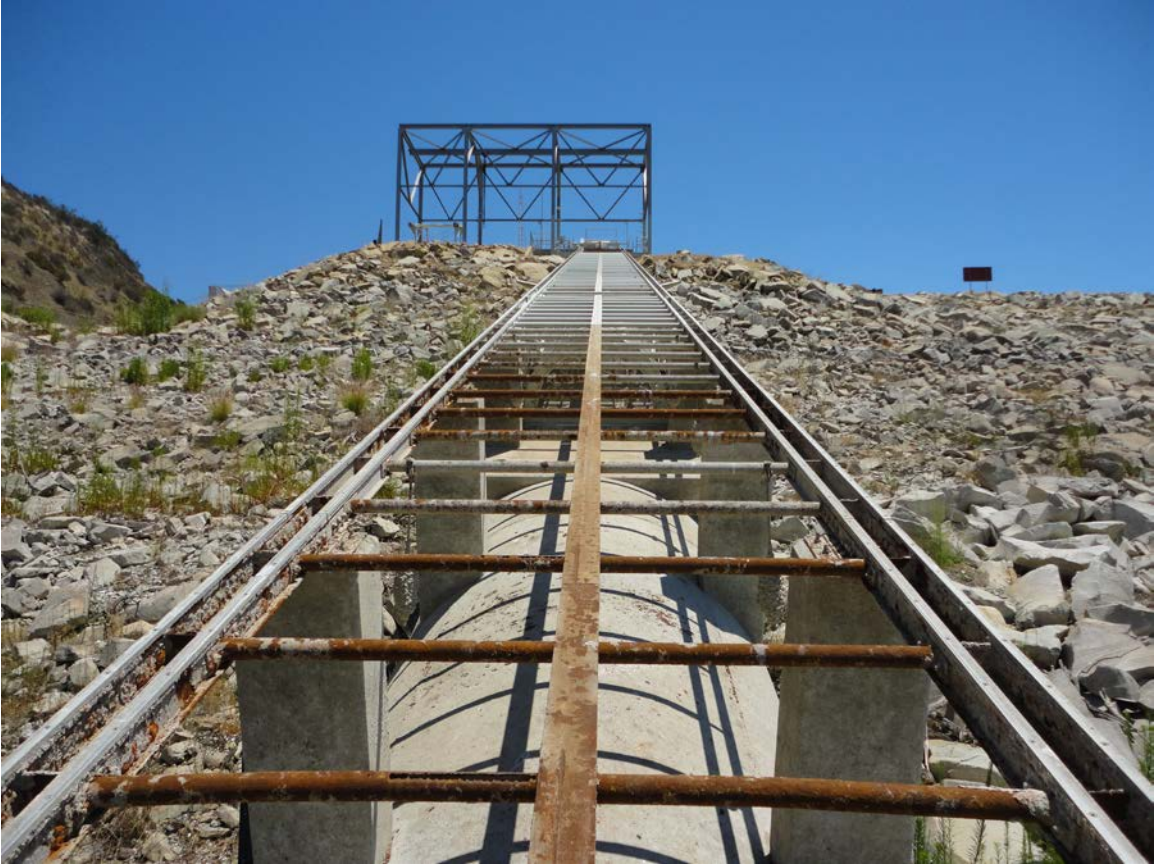
View of cross member wear
