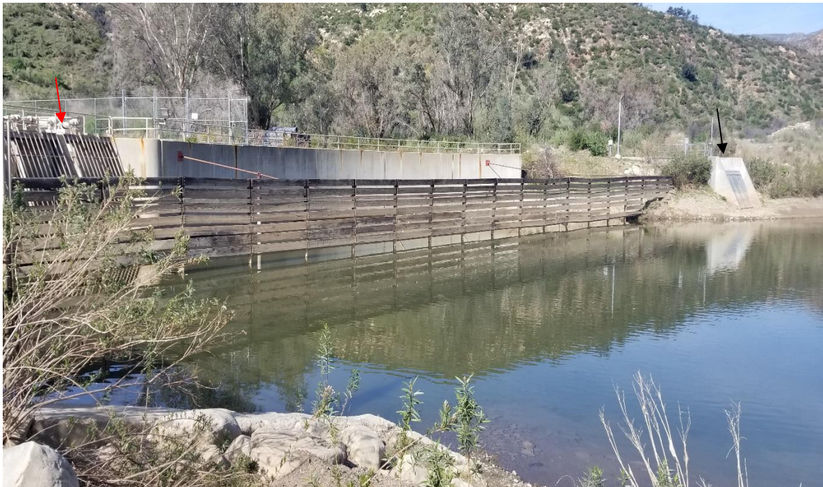
Photograph 8. View of the timber debris fence and high-flow fish exit (black arrow). The headworks is shown in back of the fence, denoted with a red arrow (February 4, 2020).
