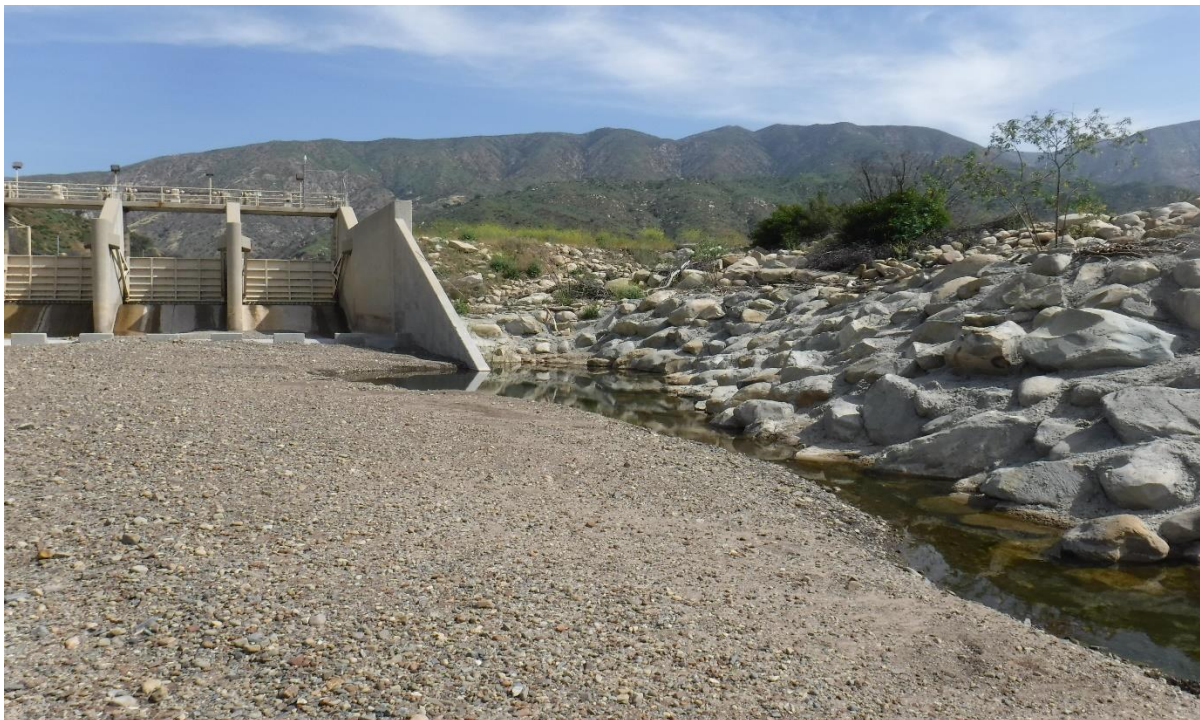
Photograph 10. View looking at the downstream side of the spillway, at the entrance pool which was completely filled in with sediment following storms post-Thomas Fire (May 2, 2019).
