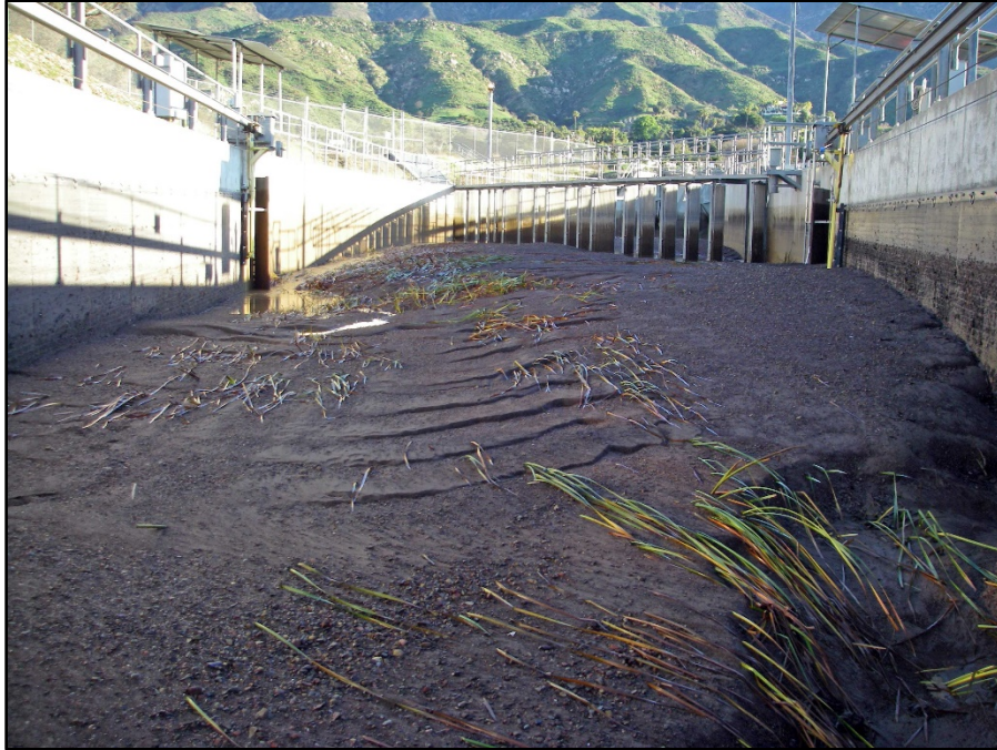
Photo 13- Sediment inundation in Robles Diversion screenbay prior to emergency cleanout
