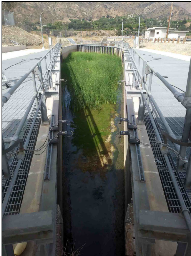
Photo 12- Dense vegetation and sediment deposition in Robles Diversion screenbay
