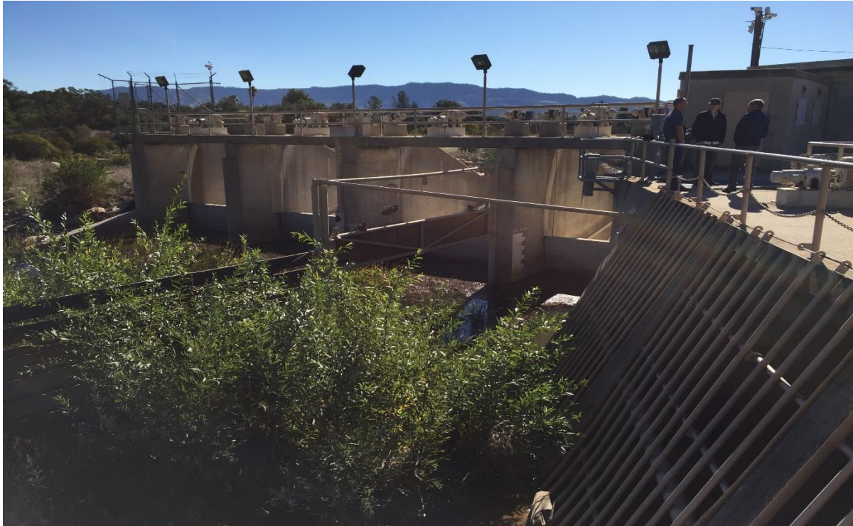
Photograph 7. View of upstream side of the spillway, radial gates and headworks (December 13, 2019).
