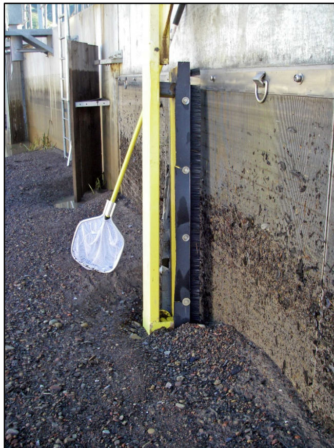
Photo 14- Sediment inundating fish screens and brushes in Robles Diversion screenbay
