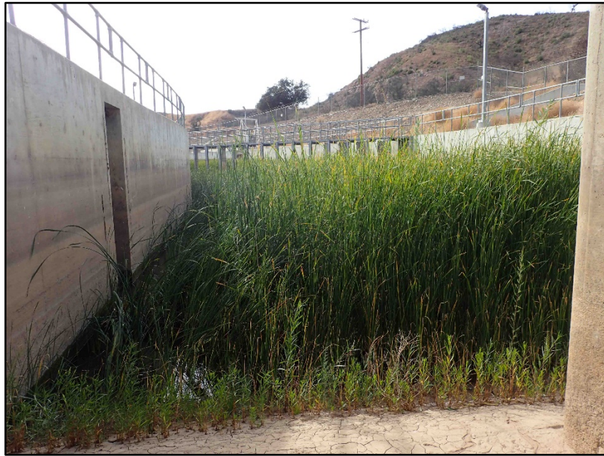
Photo 11- Dense vegetation and sediment deposition in Robles Diversion screenbay
