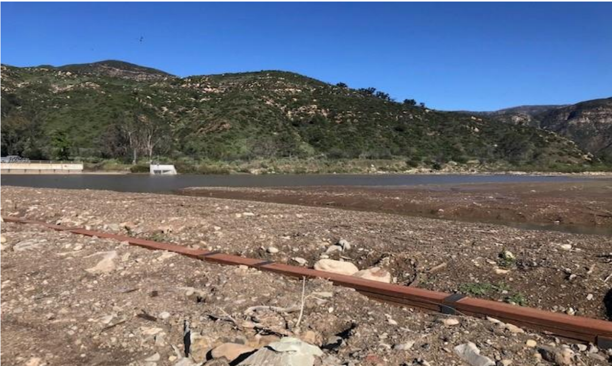
Photograph 2. View of the timber cut-off wall after repairs to the wall were made in November 2019. Light vehicles can drive over the timber cut-off wall to access the fish passage facility to the west, without driving through the active flowing channel (February 2, 2020).
