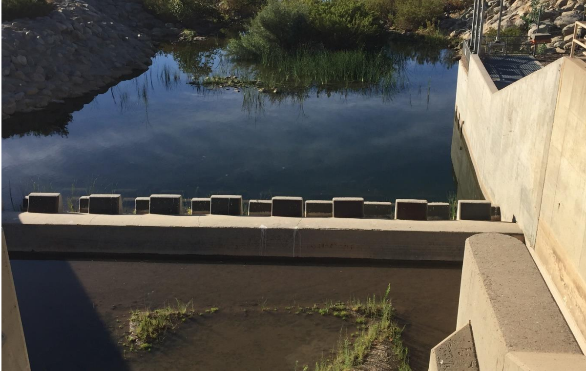
Photograph 9. View of the baffled apron downstream of the spillway, at the beginning of the entrance pool (December 13, 2019).
