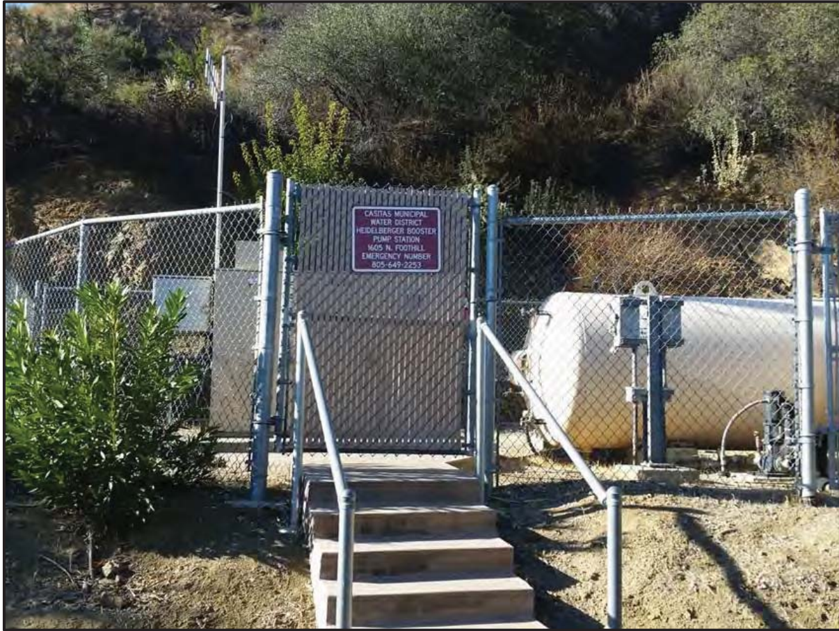
Photograph 3 Heidelberg Booster Pump Station
