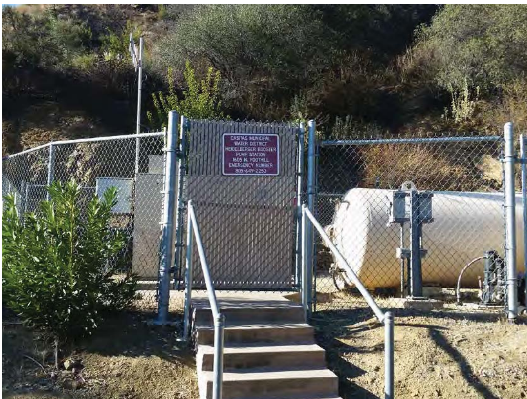
Photo 2. Heidelberg Booster Pump Station, facing west
