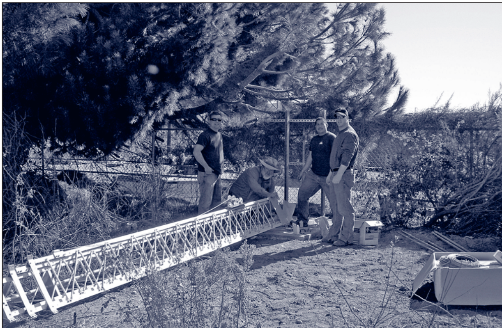
From left: Casitas employees John Parlee, Gerry Herrera, Kevin Champlin and Troy Legg, a consultant with Electronic Systems Technology, work on installing one of two radio towers that make up part of Casitas' new wireless communication system.
