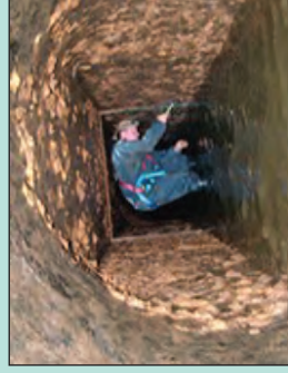
Scott MacDonald performing maintenance on 4'x4' emergency gate guides deep inside dam's outlet works.
