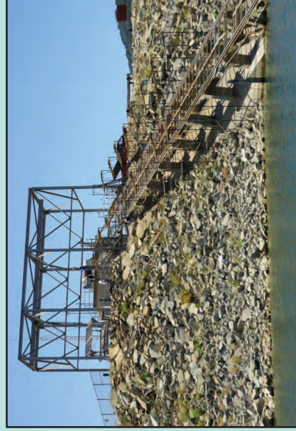
Setting up scaffolding for recoating of dam's hoist house equipment and intake track.
