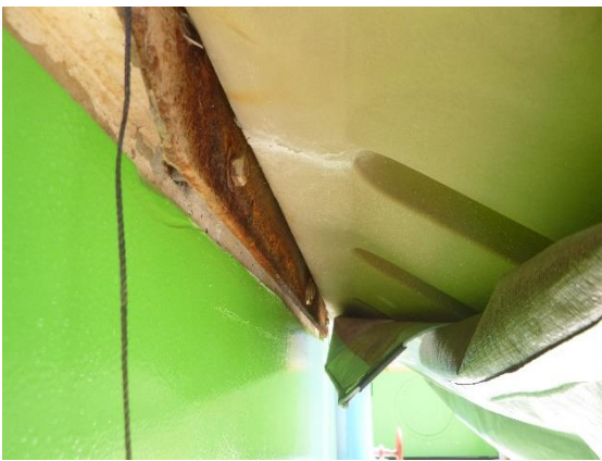
Fig 1.23. Corrosion on slide support
