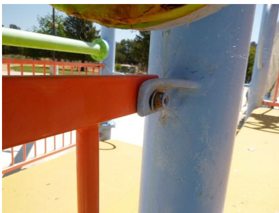
Fig 1.41. Corrosion on railing bolt connection
