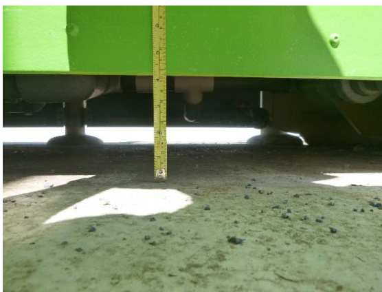
Fig 1.17. Gap at base of structure
