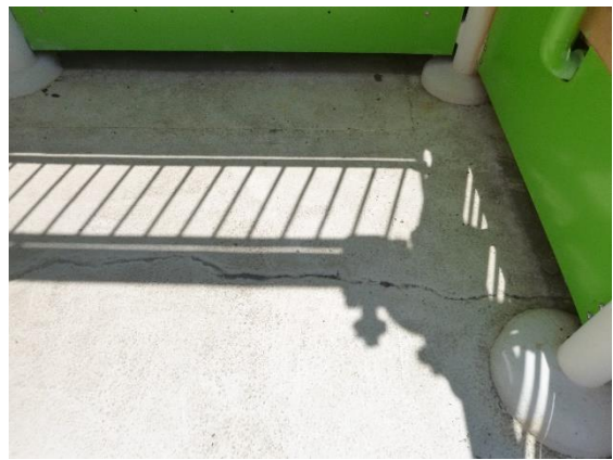
Fig 1.24. Crack in pool floor
