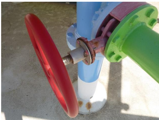
Fig 1.5. Steering wheel joint corrosion
