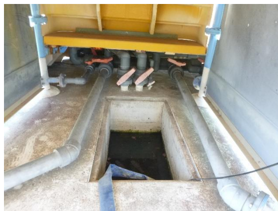
Fig 1.42. Play feature piping
