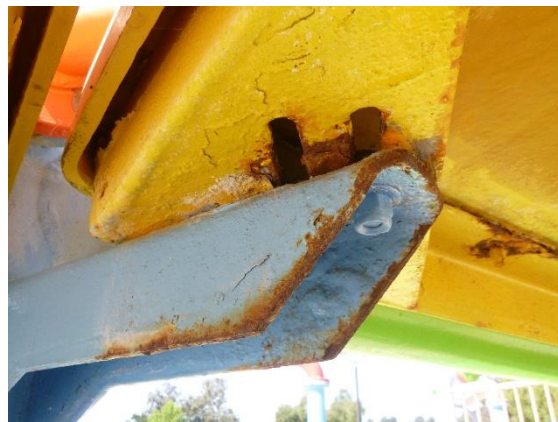
Fig 1.6. Corrosion underneath platforms
