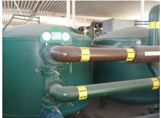
Fig 1.26. Play structure filtration
