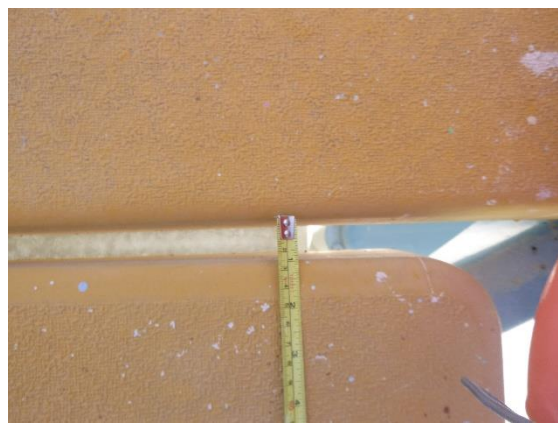
Fig 1.18 Gaps in platform connections
