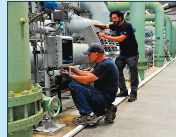
Operations and Maintenance staff work diligently to ensure high water quality at the Marion R. Walker Treatment Plant near Lake Casitas, CA.
