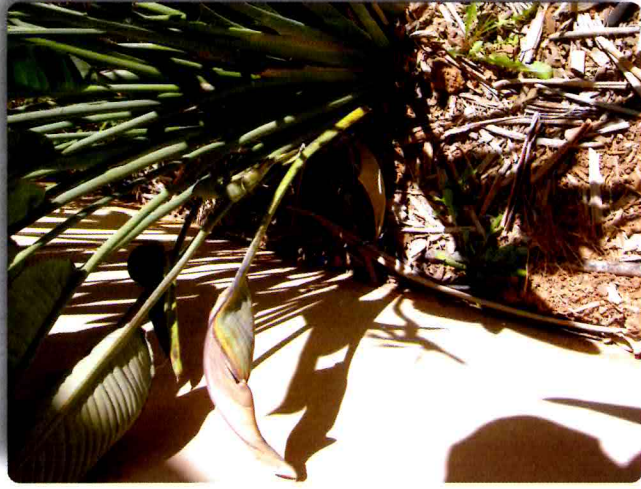
Drip line with micro-sprinkler.
