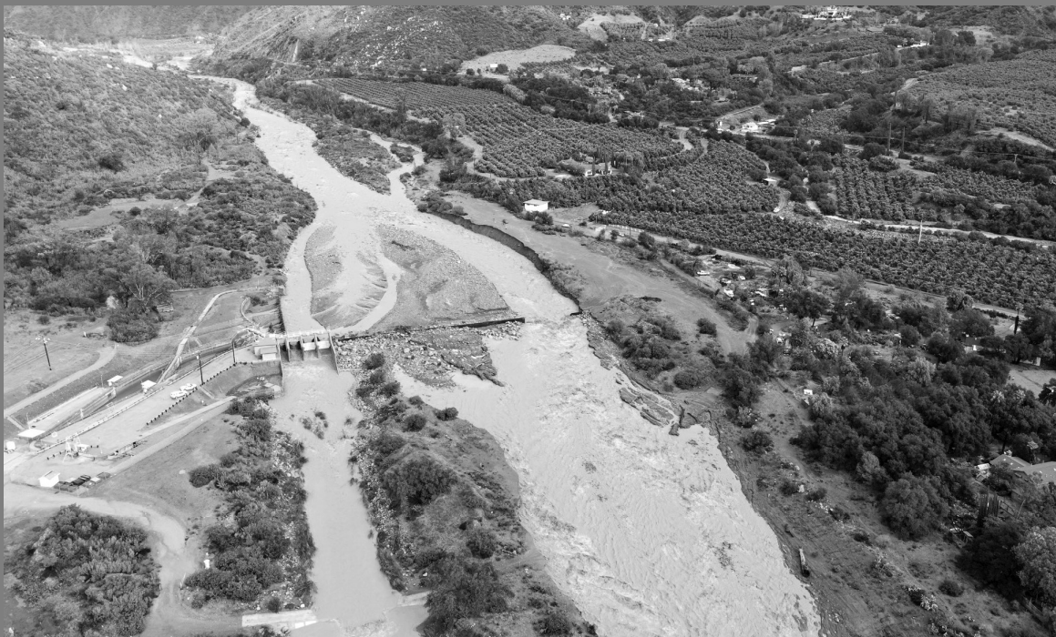
Photo above is from January 10, 2023 following the storm damage that occurred on January 9-10, 2023. The timber cutoff wall was breached on the eastern side causing flows to go around the diversion and fish passage structures, and the facility was filled with sediment and debris.
