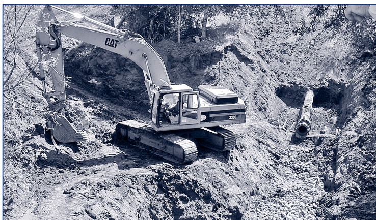
Casitas' staff and contractors worked to remove old pipeline and prepare to replace it.
