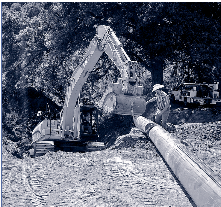
Contractors and Casitas' pipeline crew replaced a section of deteriorating steel pipe with a high density polyethylene pipe.
