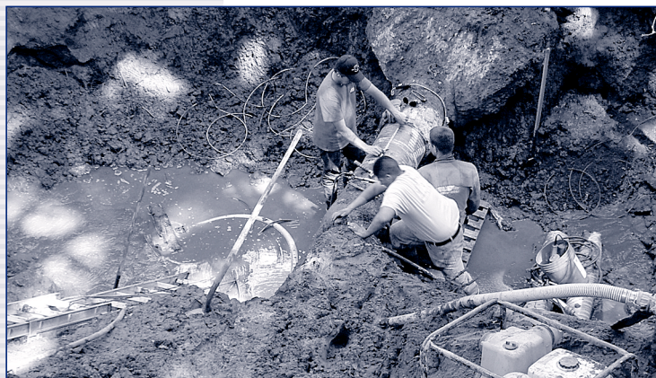
Casitas workers at pipeline break, where they worked nearly non-stop for two days.
